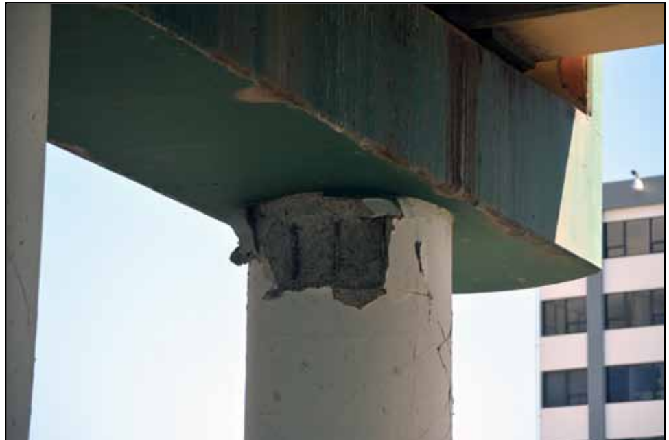
Damage to a new column.
