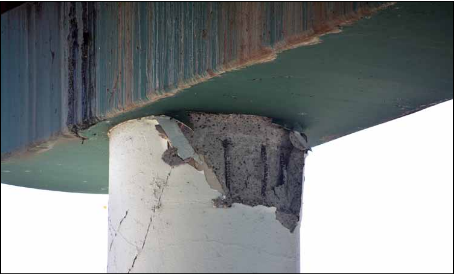
Damages to original construction's columns.
